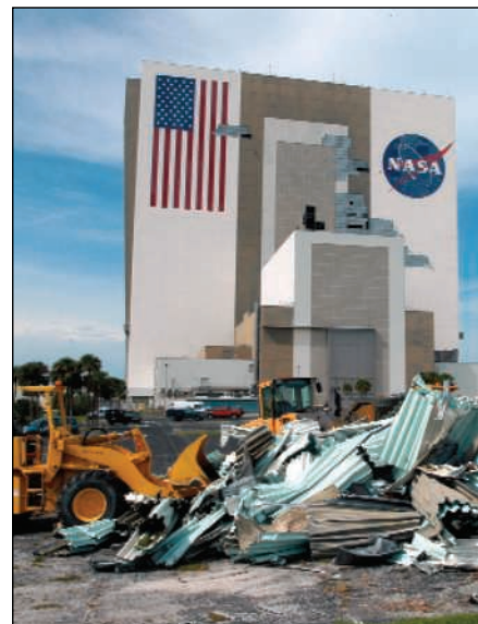
Space scuttle. Hurricane Frances shredded the walls of a Kennedy Space Center building used to assemble shuttle parts.
